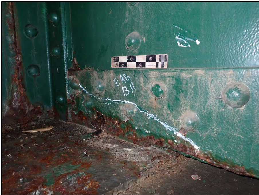
Photo 12 – Looking east at north web of beam 11 at the east abutment exhibits a 14" long x 4" tall area of up to 1/16" deep painted over section loss in the bottom of the web plate.
