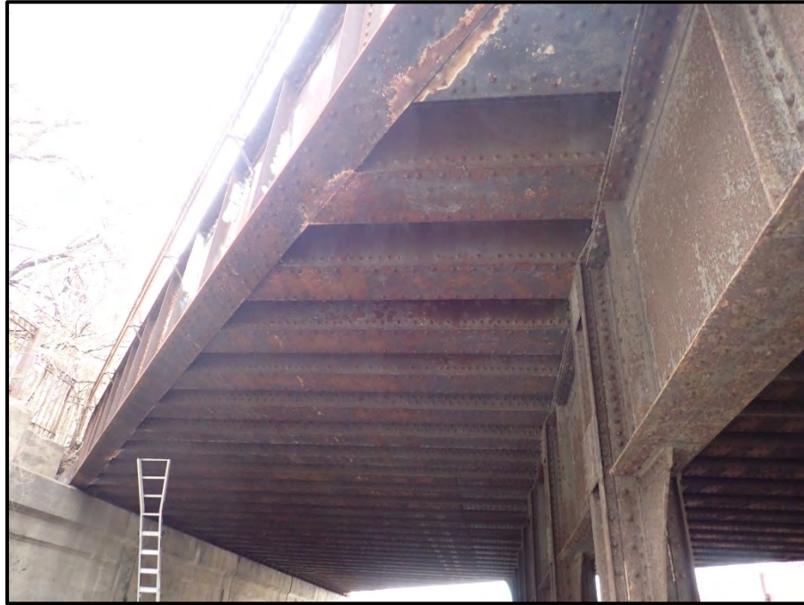
Photo 5 – Looking north at the underside of span 1. Note: moderate surface rust throughout with isolated locations of section loss.
