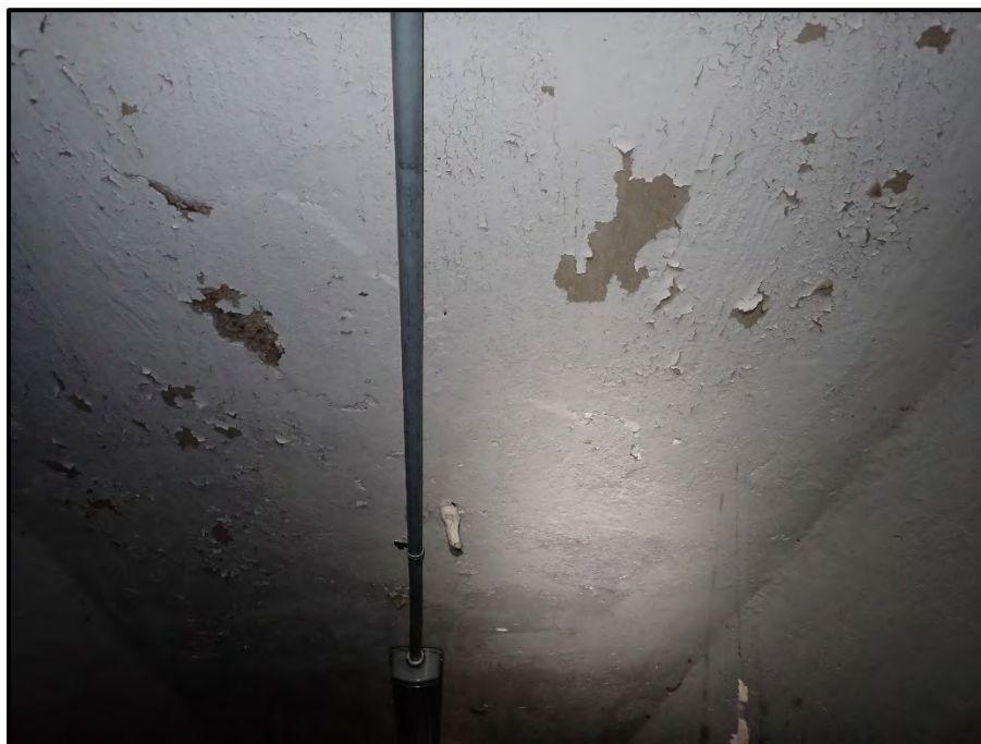
Photo 13 – Looking north at 2 SF of delaminations, 52' from the north end of the tunnel.
