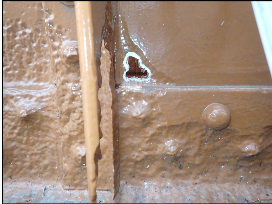
Photo 13 – Looking south at outboard face of girder 1 adjacent to 3rd stiffener from end. Note: 1 1/4" painted over corrosion hole on web.
