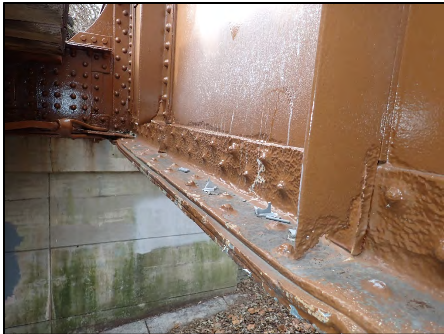
Photo 18 – Looking northwest at the inboard face of girder 1. Note: Inboard face of girder 1 bottom flange angle. 1/8" average, 3/8" max painted over pitting along bottom flange angle. All bottom flange angle rivets exhibit painted over section loss, half of which are 50% or greater.
