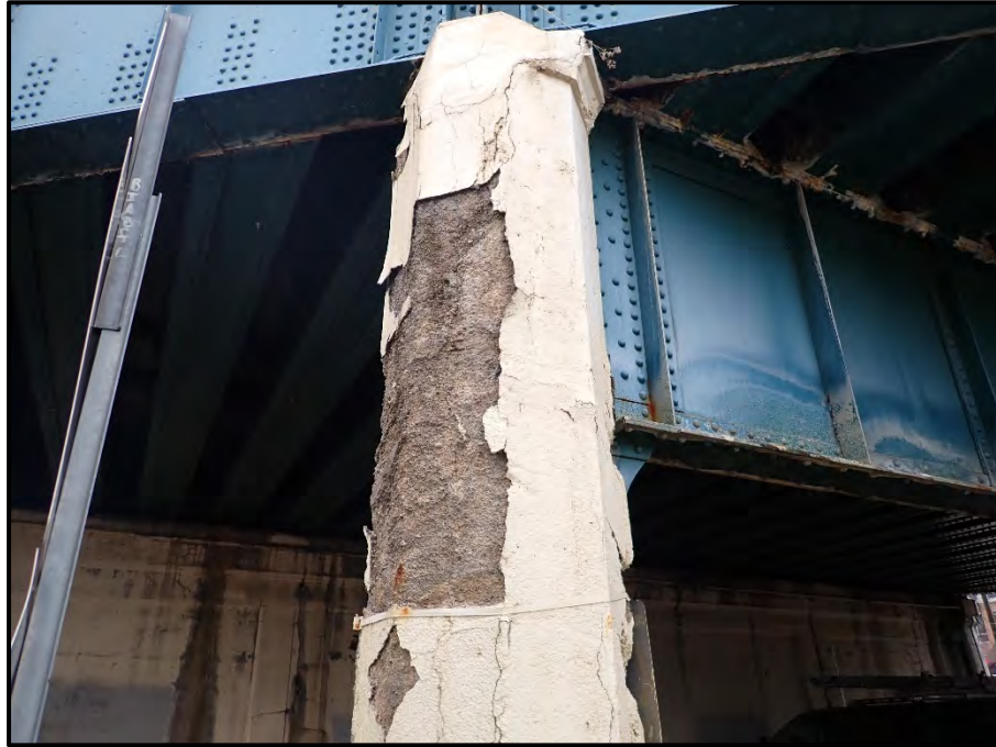
Photo 15 – Looking west at overall of the top half of column 7. Note: concrete is in poor condition and appears to not contain any reinforcement and only appears to protect the underlying built up steel column.
