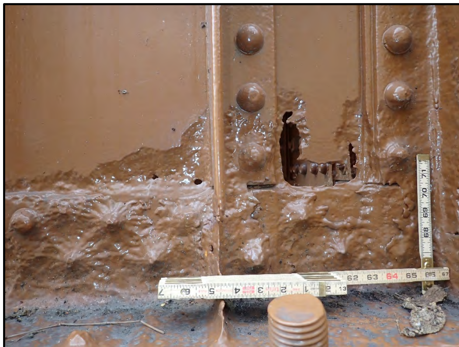
Photo 12 – Looking south at outboard face of girder 1 at the west abutment. Note: 4" x 4" painted over through hole in web plate between the first and second web stiffener from the end.
