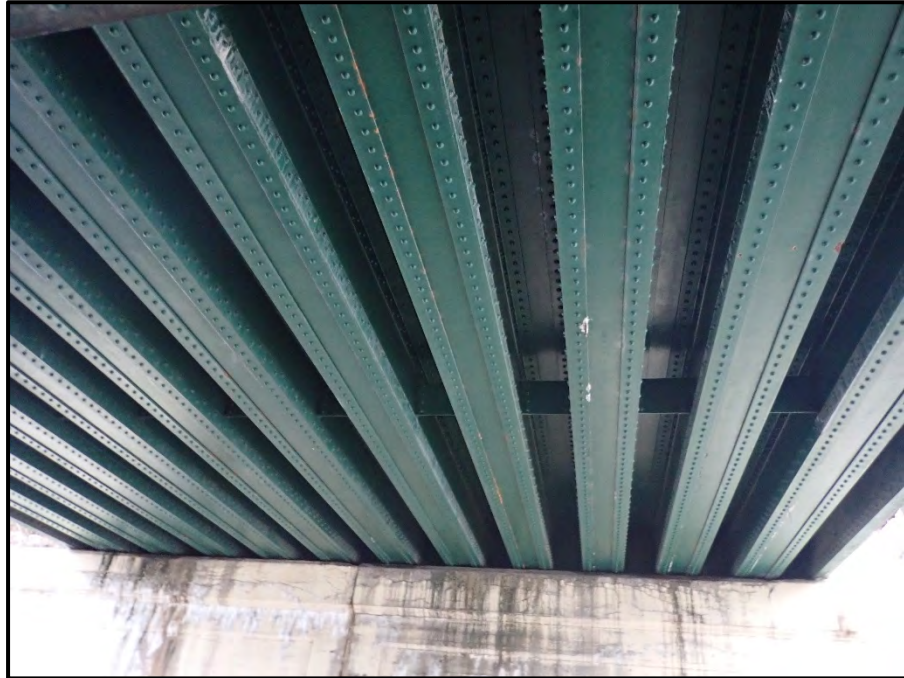
Photo 5 – Looking west at the underside of span 1. Note: isolated locations of surface corrosion with minor section loss.
