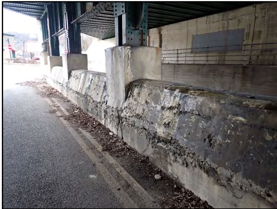
Photo 12 – Looking northeast at an overall view of the partial height pier wall at column 4. Note: the pier wall exhibits heavy deterioration intermittently, full length. The concrete encasement extensions around base of columns exhibits minor crack, but are generally in good condition.
