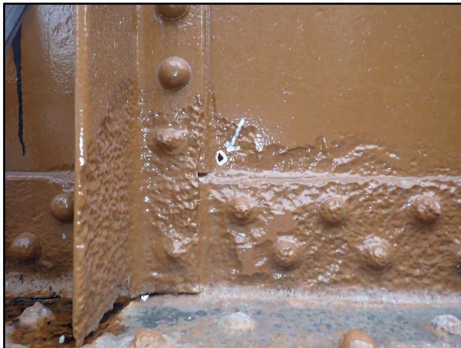
Photo 11 – Looking south at outboard face of girder 1 at east end between 3rd and 4th stiffeners from east, adjacent to 4th stiffener. Note: 1/2" diameter corrosion hole through web with adjacent 1/8" deep painted over pitting.
