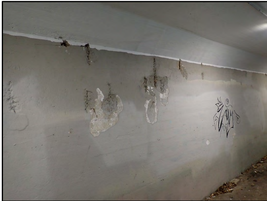
Photo 10 – Looking northwest at 30 SF of intermittent spalling on the west wall, up to 1" deep.
