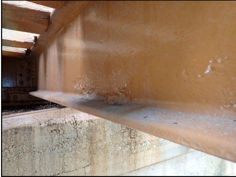
Photo 19 – Looking southwest at stringer 3 in floor beam bay 2-3. Note: Widespread 1/16" deep painted over pitting along bottom 4" of web.
