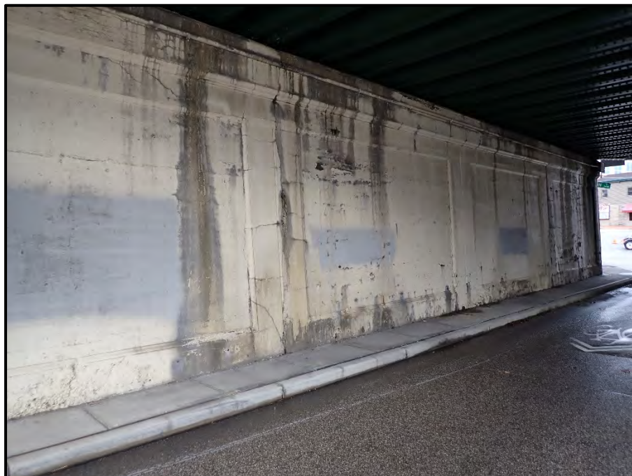
Photo 8 – Looking northwest overall elevation of the west abutment exhibits vertical and horizontal moderate width cracks in cap. Cracking is heaviest in south half of abutment.
