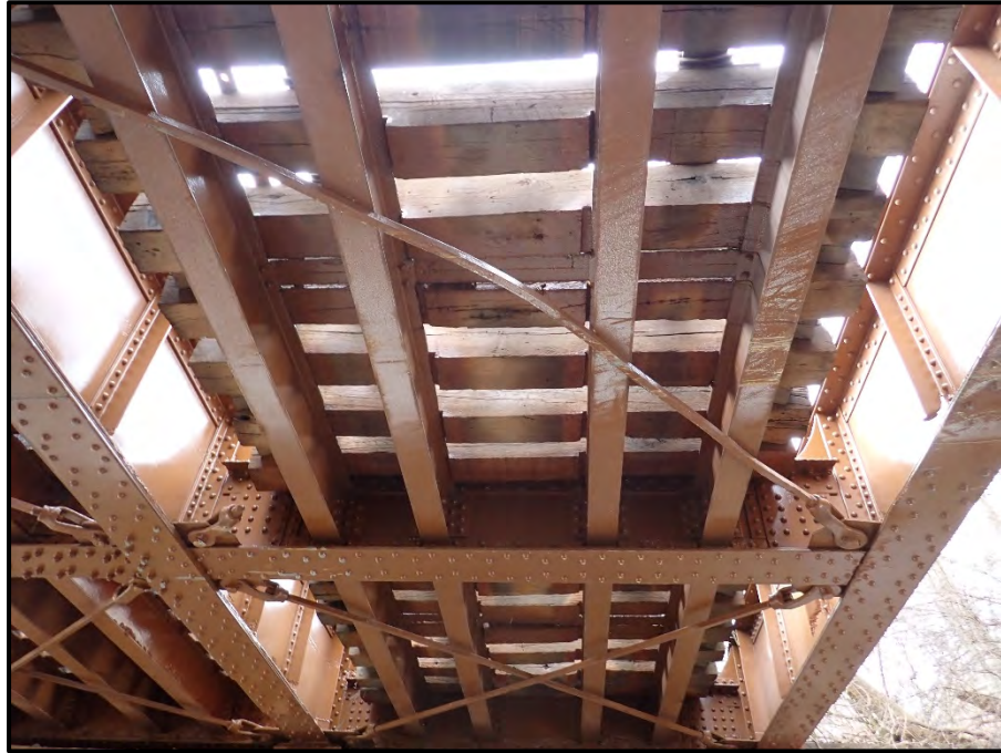
Photo 5 – Looking west at the typical underside between girders 1 and 2. Note: one missing and one bent lower lateral bracing bar.
