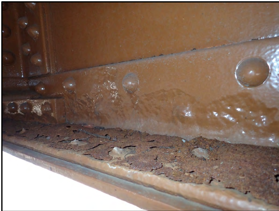
Photo 20 – Looking southwest at East face of floor beam 2 between stringers 2 and 3. Note: Typical 1/16" deep painted over pitting along bottom 4" of web and bottom flange angles.
