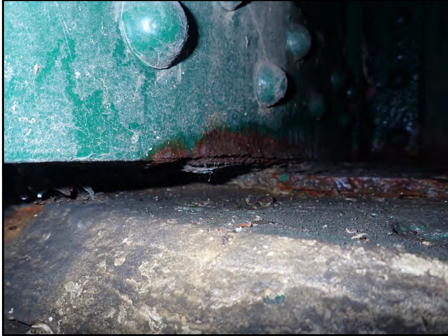
Photo 11 – Looking east at underside of beam 3 at the east abutment. Note: minor surface corrosion and water staining on the bottom of beam with negligible section loss.
