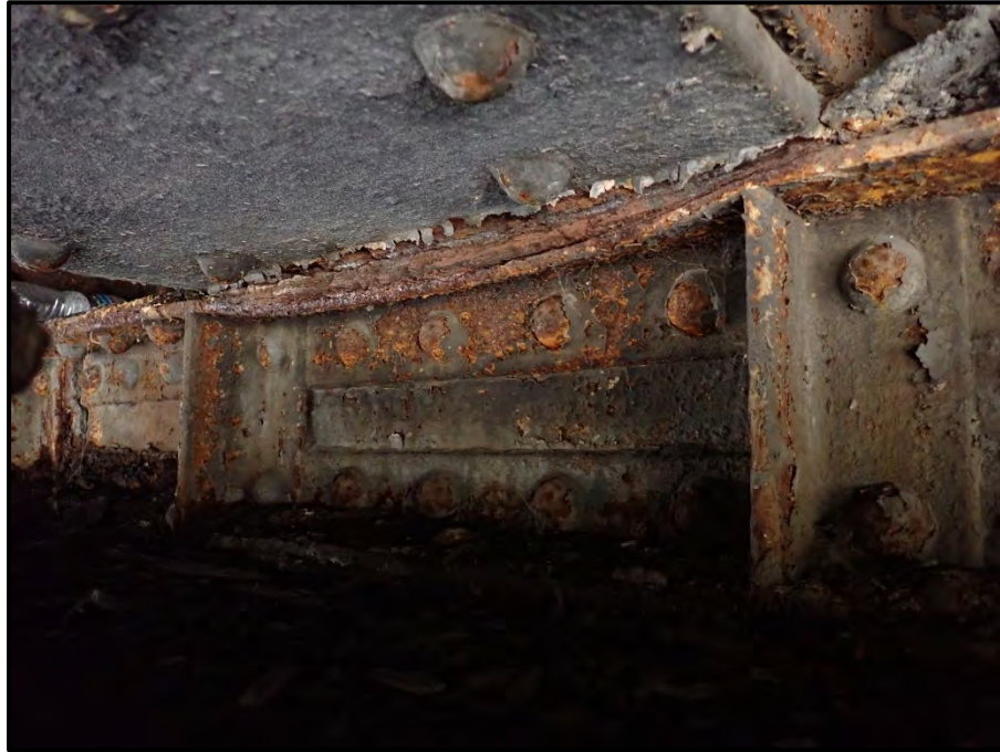
Photo 11 – Looking west at west abutment steel bearing seat under floor beam 15. Note: pack rust up to 1" thick causing deformation to bottom flange
