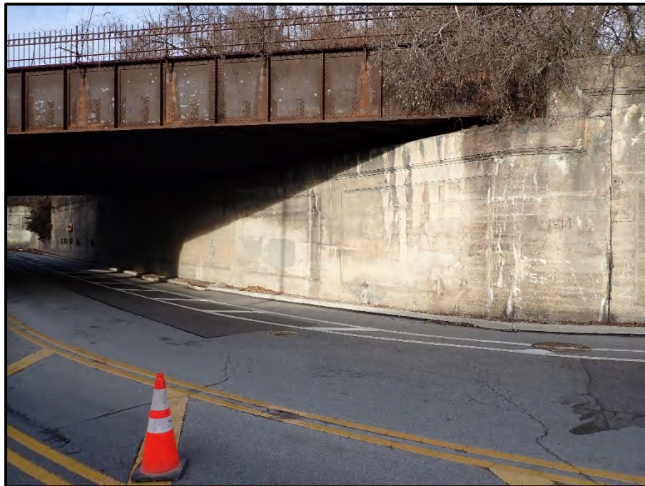
Photo 6 – Looking northeast at the west abutment elevation. Note: some minor to moderate width cracks to the abutment wall. Cracking is heaviest in the cap directly under the bearing seat.
