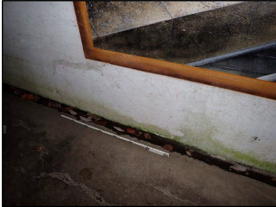
Photo 11 – Looking west at 3.5' x 1' delamination on the west wall 10' from the north end of the tunnel.
