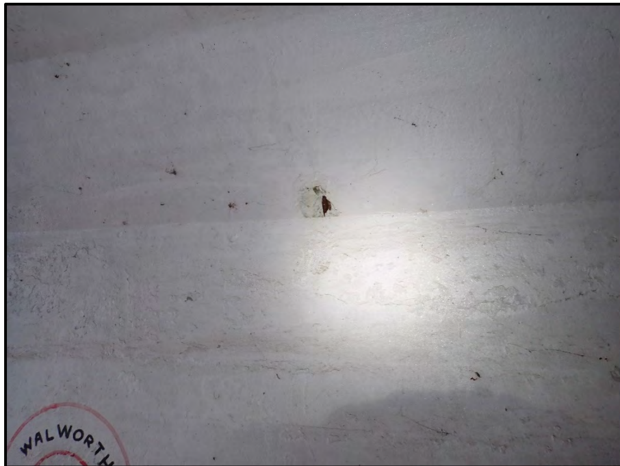
Photo 12 – Looking west at 4" diameter x 1/2" deep spall 10' from the south end of the tunnel.
