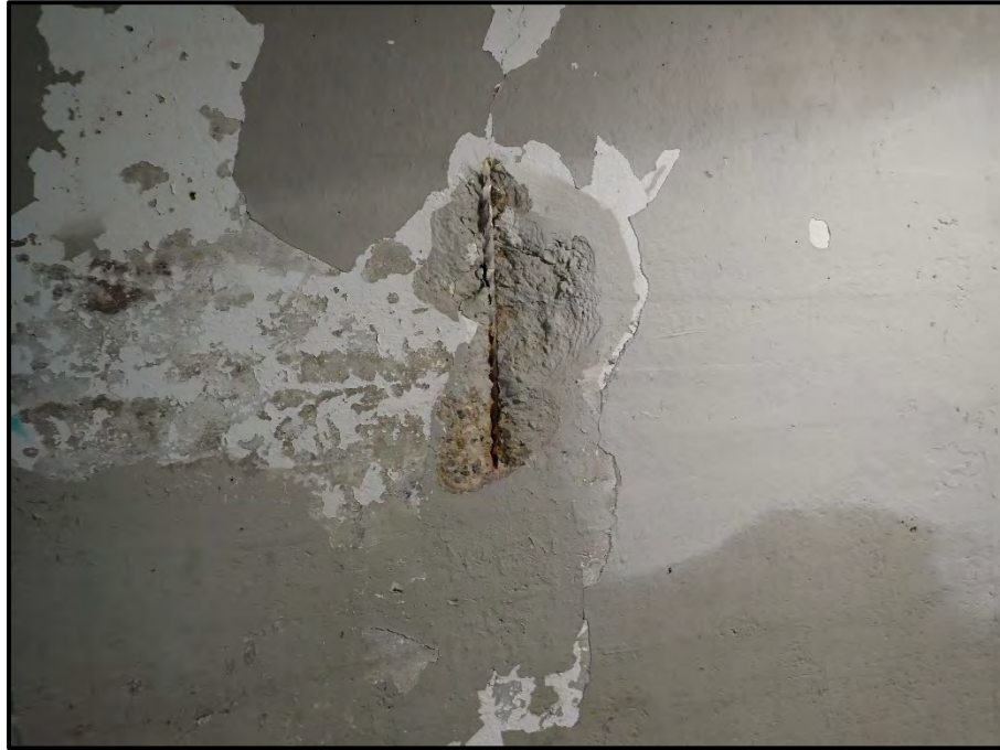
Photo 15 – Looking west at 2' x 1' x 1" deep spall with one exposed and corroding spiral bar on the west wall, 8' from the south end.
