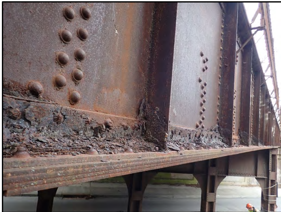
Photo 10 – Looking southwest at girder 1, east end. Note: heavy laminating corrosion and corrosion holes through bottom of outboard vertical stiffeners. First 3 stiffeners from end exhibit corrosion holes up to 5" tall, full width.
