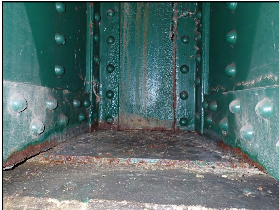
Photo 10 – Looking east at typical bearing seat condition between beams 3 and 4 and the east abutment. Note: minor surface corrosion, water staining, and active leakage at bearing seat with negligible section loss.
