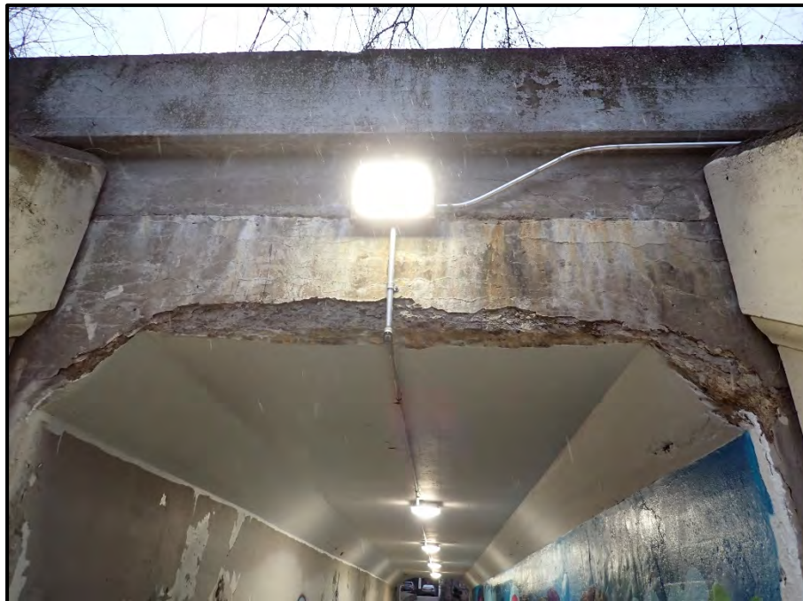
Photo 6 – Looking north at full width (8') x 6" tall x up to 1" deep spall in the bottom corner of the south end tunnel entrance. 1' tall x 8' wide area of adjacent delamination above spall.
