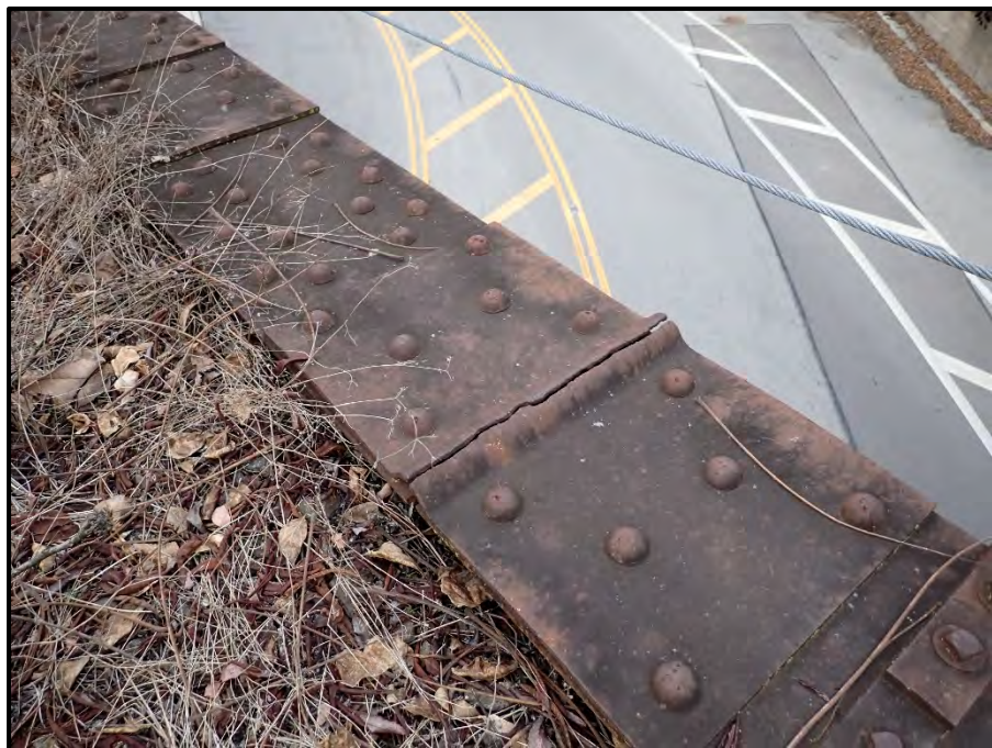
Photo 14 – Looking northwest at top flange strap/splice plate at midspan of girder 1. Note: full width crack in plate. Similar at same location, girder 2. Appears intentional.
