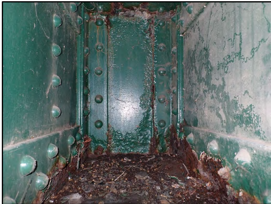
Photo 14 – Looking east at Overall of the steel backwall between beam 12 and 13 at the east abutment. Note: up to 1/8" painted over section loss throughout with a 4" wide x 1" tall void/corrosion hole in the top of the back and end of deck pan. Ballast is exposed.
