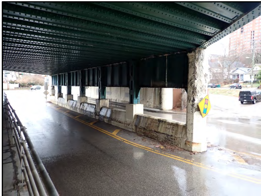
Photo 6 – Looking northwest at the east face of the pier. Note: heavy spalling on column 7 and along the concrete pier protection.
