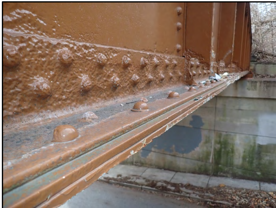
Photo 16 – Looking southwest at the outboard face of girder 1 bottom flange angle at east half of girder. Note: 1/8" average, 3/8" max painted over pitting along bottom flange angle. All bottom flange angle rivets exhibit painted over section loss, half of which are 50% or greater.
