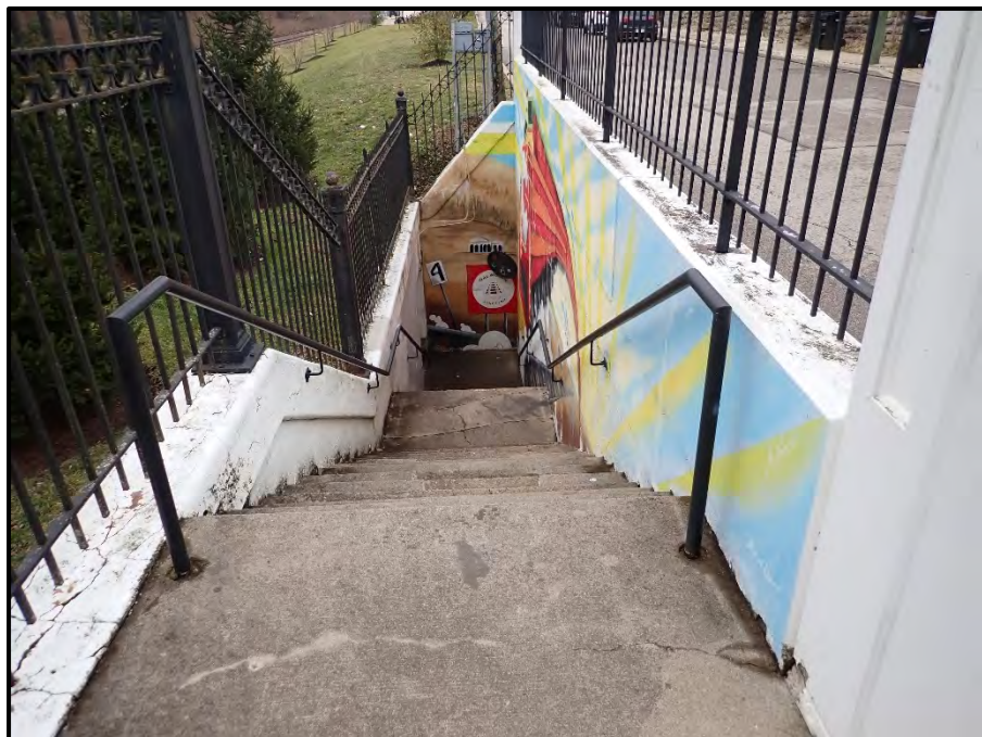
Photo 8 – Looking west down the north end steps. Note: minor isolated crack in the concrete steps. Flaking seal coat and insignificant width isolated cracks in retaining walls.
