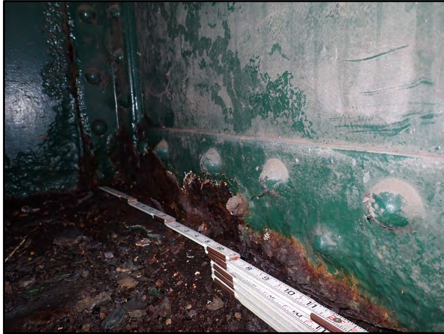
Photo 13 – Looking east at the north face of beam 13 bottom of web at the east abutment a 15" long x 3" tall area of active corrosion with up to 1/16" deep section loss.
