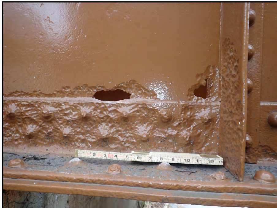
Photo 10 – Looking southeast at the outboard face of girder 1 at east end between the 2nd and 3rd stiffeners from east. Note: 4 1/2" x 1 1/2" and 2 1/2" x 1 1/2" through hole in web plate with adjacent pitting down to knife edge.
