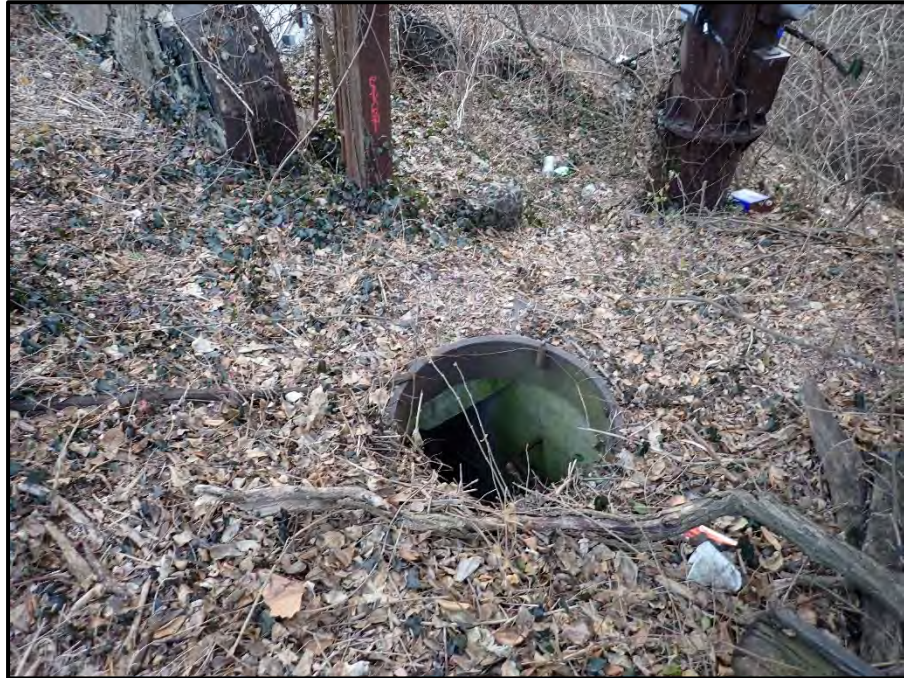
Photo 13 – Looking south at the open manhole at the southwest approach.
