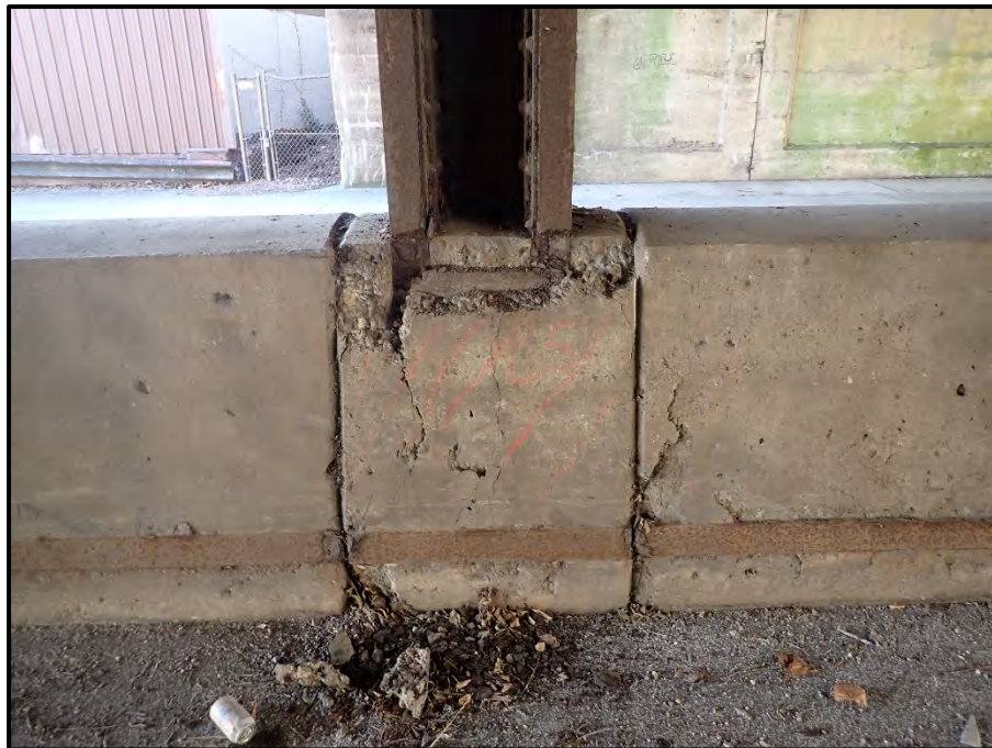
Photo 8 – Looking west at an overall of the east face vertical angle legs at the pier wall exhibit up to 75% section loss to angle legs over a 1" tall x full width area.
