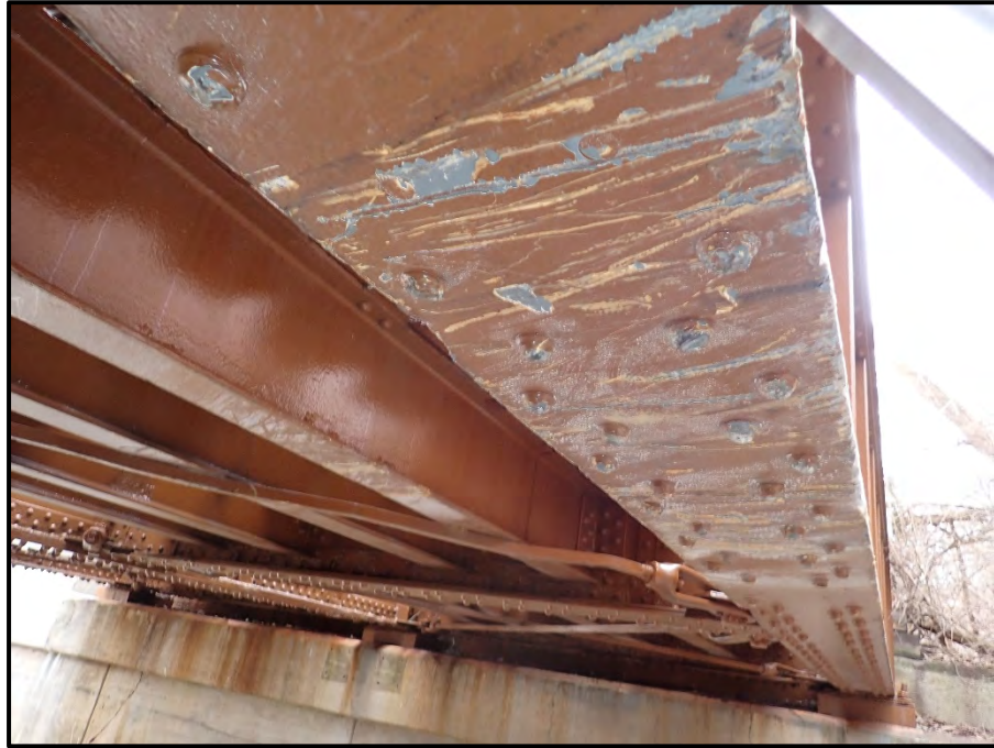
Photo 17 – Looking west at the bottom flange of girder near mid-span. Note: Multiple impact scrapes and gouges along bottom flange plates. Minor deformation of bottom flange.
