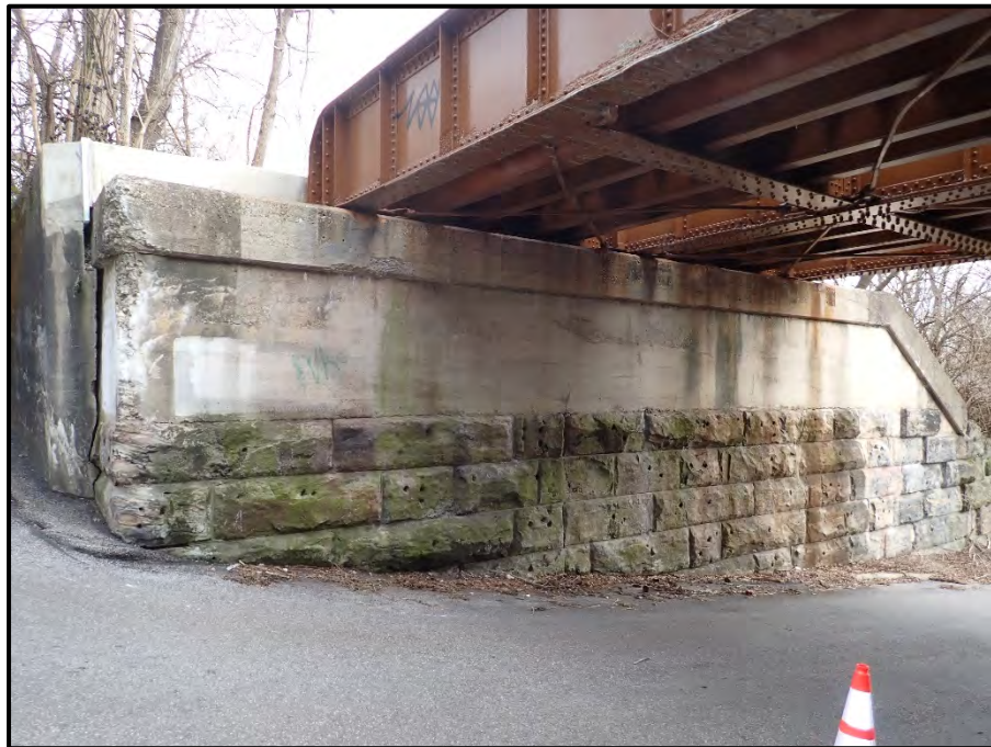
Photo 6 – Looking southeast at the east abutment. Note: moderate abrasion on the north end of the east abutment. Multiple moderate width horizontal cracks in the north end with minor efflorescence.
