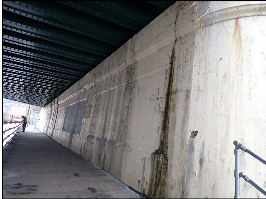
Photo 7 – Looking northeast at overall elevation of the east abutment from south end. Note: isolated delaminations totally less than 20 SF. Horizontal and vertical moderate width cracking throughout abutment cap. Concreted is generally sound around cracks.
