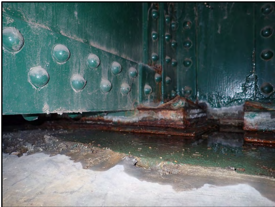
Photo 10 – Looking west at south face of floorbeam 41 bearing at the west abutment exhibits pack rust peeling the horizontal angle leg with adjacent surface corrosion with negligible section loss.
