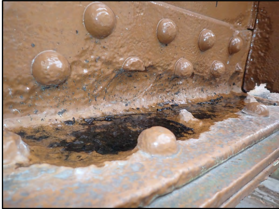
Photo 15 – Looking southeast at the outboard face of girder 1 bottom flange angle at east half of girder. Note: 1/8" average, 3/8" max painted over pitting along bottom flange angle. All bottom flange angle rivets exhibit painted over section loss, half of which are 50% or greater.
