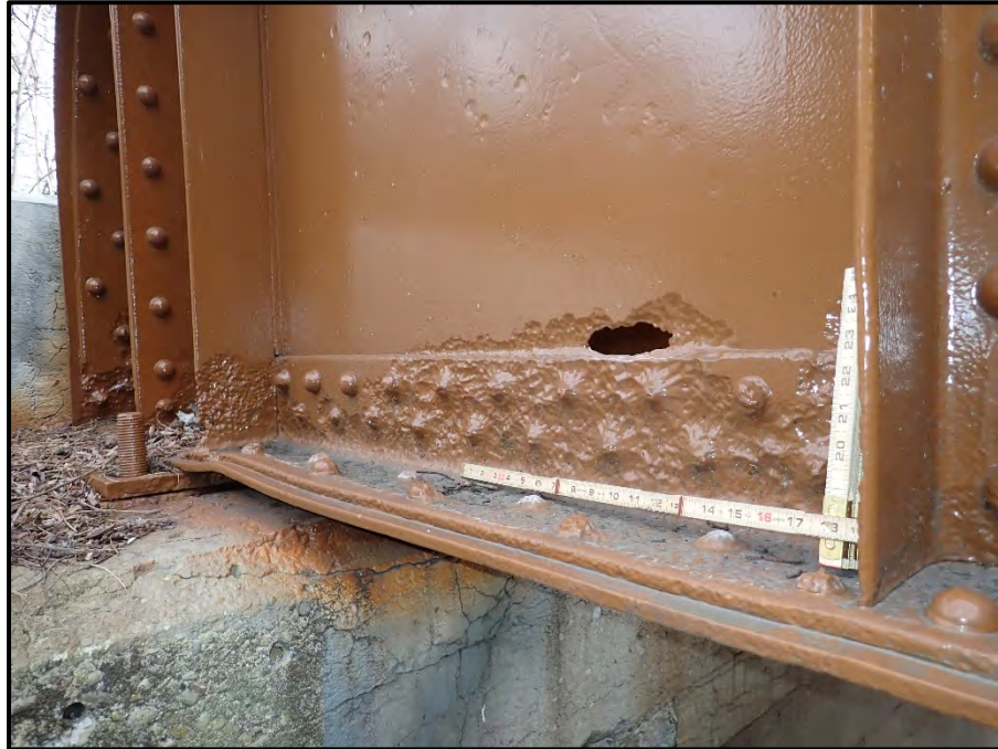
Photo 9 – Looking southeast at the outboard face of girder 1 at east end between the 2nd and 3rd stiffeners from east. Note: 4 1/2 inch x 1 1/2-inch and 2 1/2 inches x 1 1/2 inch through hole in web plate with adjacent pitting down to knife edge.
