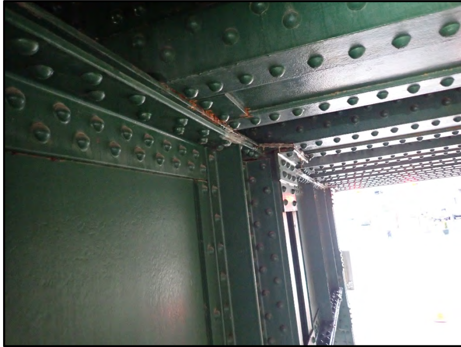
Photo 9 – Looking north at typical beam to bearing seat condition at pier 1. Photo from beam 9. Leakage is intermittent and heaviest in the end 4 beam bays.
