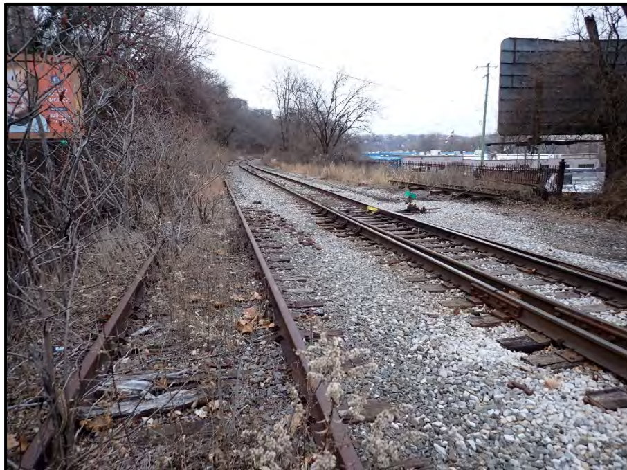
Photo 4 – Looking east at the typical top of rail condition. Note: checking and some splitting throughout rail road ties.
