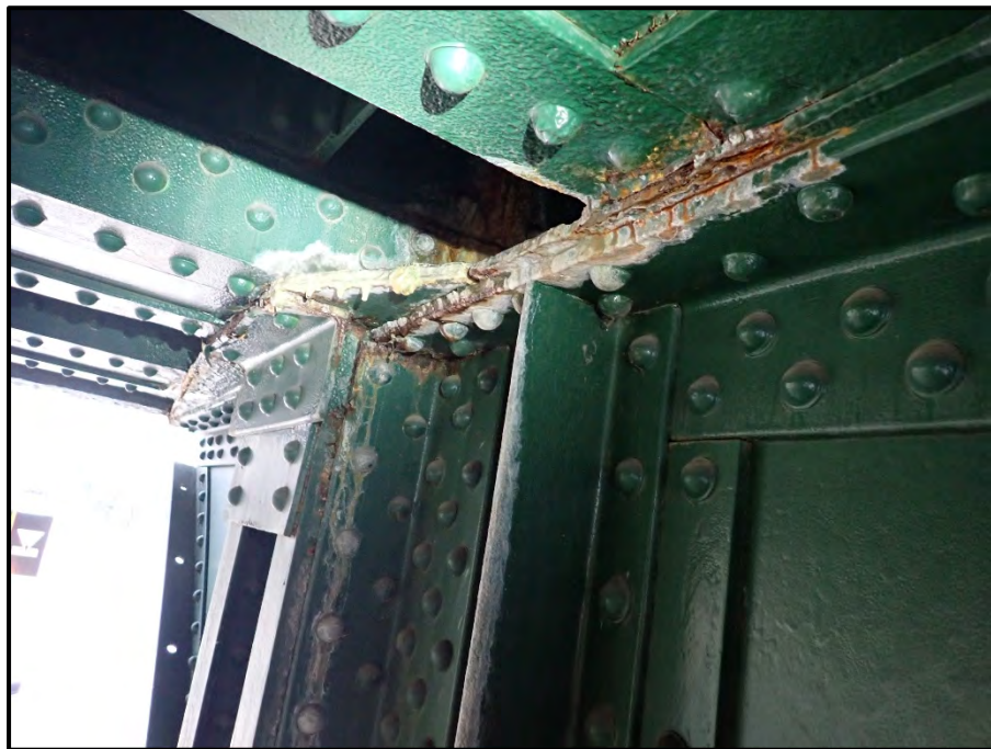
Photo 8 – Looking south at typical water leakage and moisture staining at pier 1. Note: leakage between beams 10-11 shown. Water leaks through the span 1 to span 2 deck pan interface.
