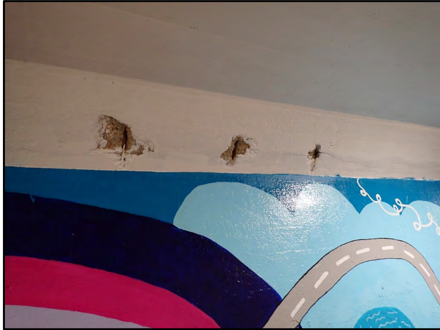
Photo 13 – Looking east at three, 1 SF spalls in the east top slab chamfer 15' from the north end with exposed and corroding rebar.
