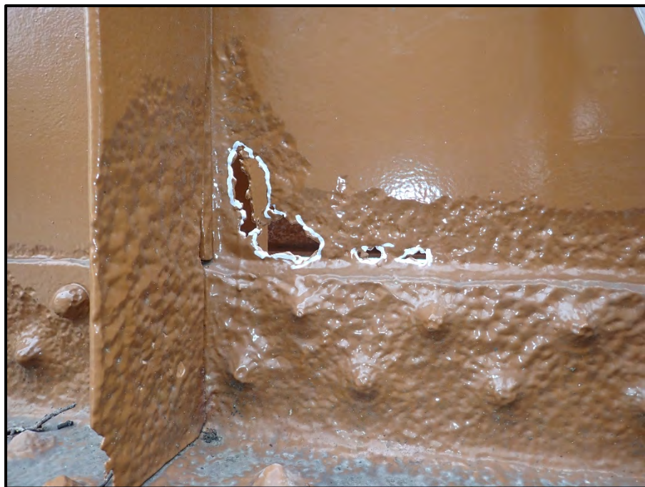
Photo 14 – Looking south at outboard face of girder 1 adjacent to 4th stiffener from west end. Note: 7" wide x up to 4" tall painted over through hole in web plate adjacent to stiffener.
