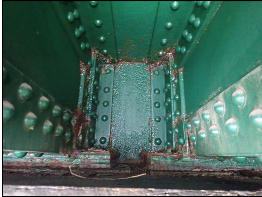
Photo 11 – Looking south a typical painted over section loss to the steel backwall between beams 7 and 8 at the east abutment. This condition is typical at multiple locations.
