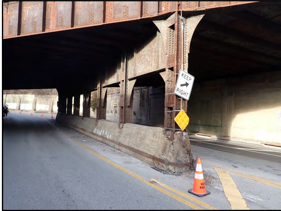
Photo 7 – Looking northeast at the west face of pier 1. Note: spalling around the base of the pier columns. Concrete repairs at the base of the columns is included in the repair plans.
