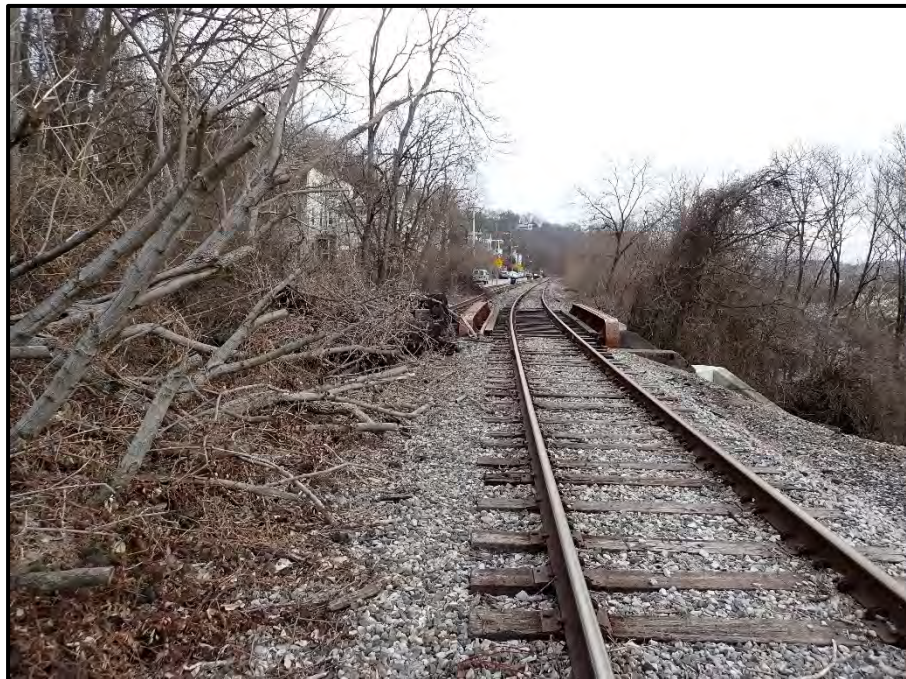
Photo 4 – End view looking east. Note: large amounts of debris and old railroad ties piled at west end.
