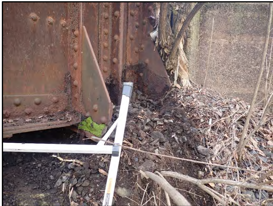
Photo 12 – Looking southwest at girder 1 at the west abutment. Note: heavy soil and debris accumulation. Active pitting, 1/16" average, to girder web and bearing stiffeners.
