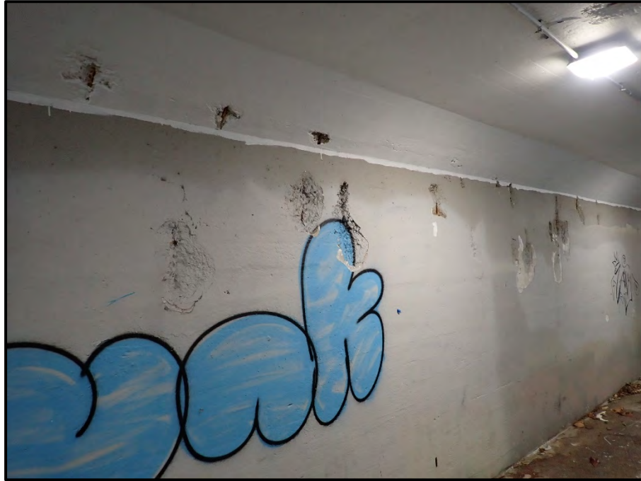
Photo 9 – Looking northwest at 30 SF of intermittent spalling on the west wall, up to 1" deep.
