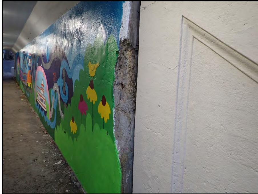
Photo 7 – Looking north at 9' x 1' x 3" deep spall in the east end of the east wall at the south entrance.
