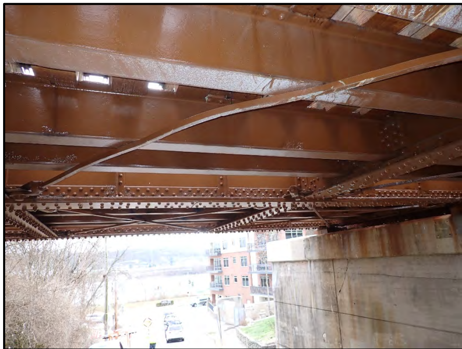
Photo 8 – Looking south at the missing lower lateral bracing bar in bays 1-2.
