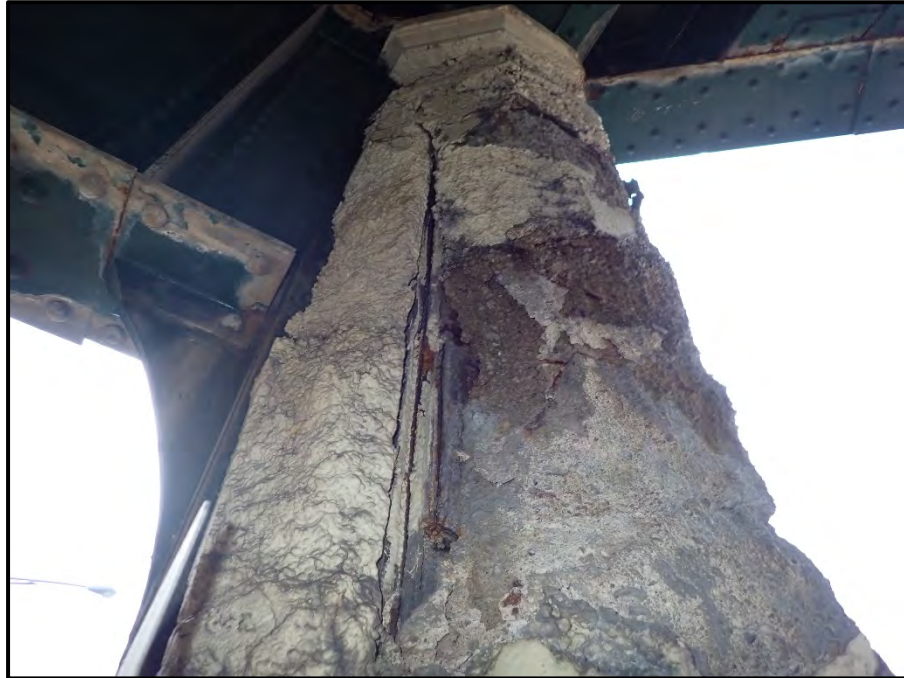
Photo 13 – Looking east at overall of column 7. Note: concrete is in poor condition and appears to not contain any reinforcement and only appears to protect the underlying built up steel column. A small portion of the steel column is exposed and is in poor condition and exhibit section loss and pack rust between components up to 1/2".
