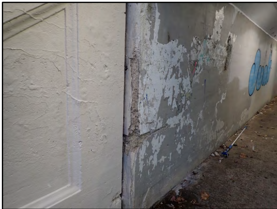
Photo 8 – Looking northwest at 3' x 6' x 2" deep spall in the south end of the east wall at the south entrance.
