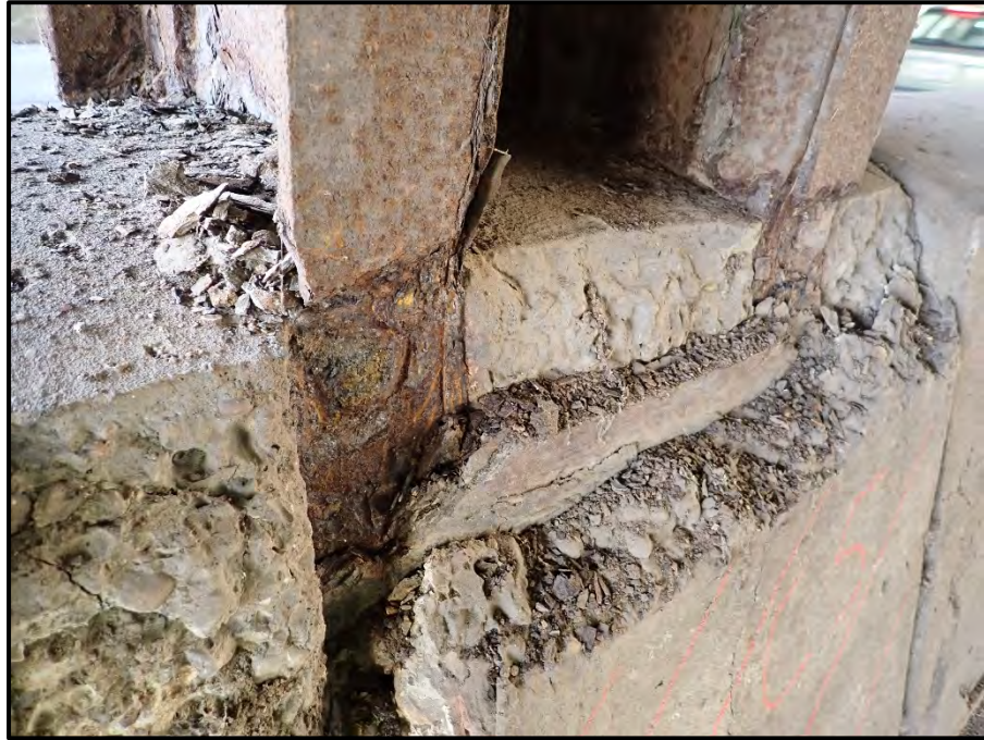
Photo 9 – Looking west at an overall of the east face vertical angle legs at the pier wall exhibit up to 75% section loss to angle legs over a 1" tall x full width area.
